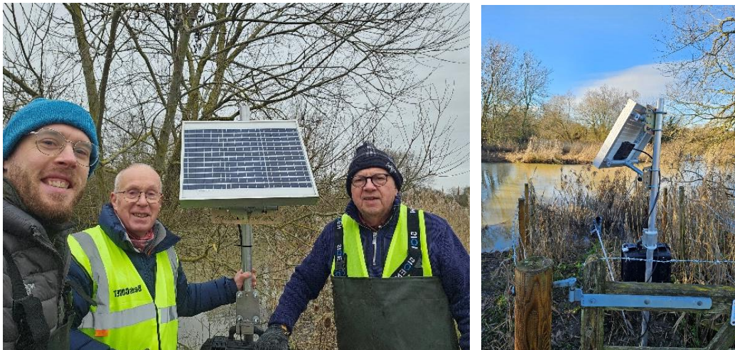
Left: Installation of site 2 (l-r: Liam from UoB, Mike & Alan from BedsGOVET). Right: downstream installation site, a standalone communication station and sonde stilling well.
